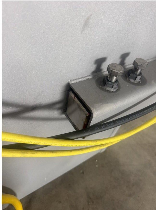
Close-up of the auger drawbar fully seated flush with the end of the receiver tube, showing two of the bolts that fasten the auger assembly to the capture tank.
